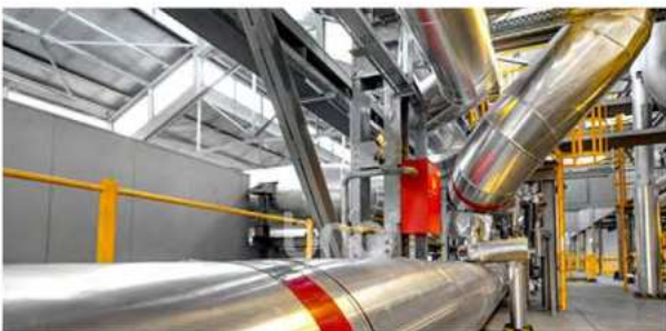
Gas Export Pipeline MAA - Ahmadi, Kuwait
